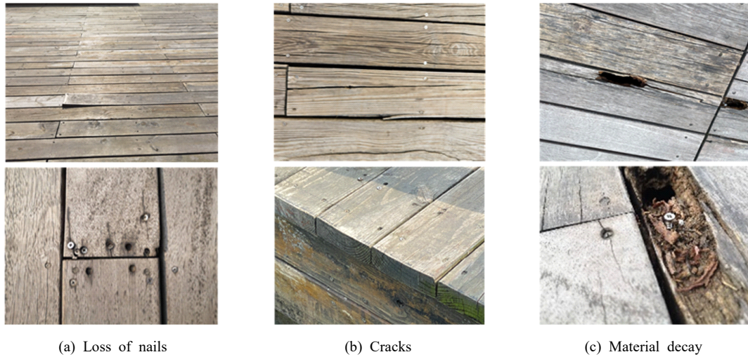
Fig. 1. Typical problems observed in timber boardwalks.
