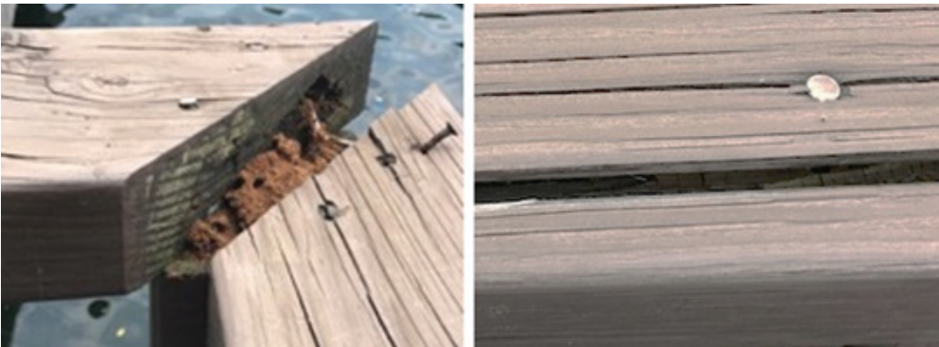
Fig. 3. The decayed parts of the cap rails.
