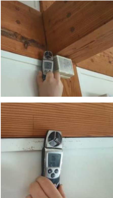
Fig. 8. Air leakage in post-beam construction.
